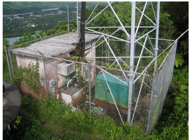
Figure 10. Cell tower and equipment shelter.
