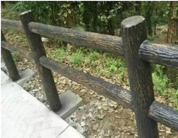
Figure 89. Example of imitation wood handrails made of concrete. 15
